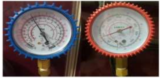
Fig. 3.3.1 Suction and Discharge pressure gauges
