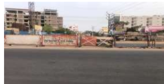
Figure 4.5: At chainage 2.600 Km, Barricades provided are damaged. Need to be replaced
